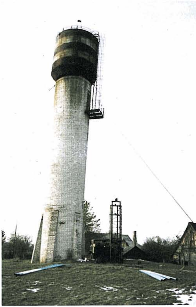
Fig. 4. The tilted water-supply tower in Kirdonys village, Biržai district
