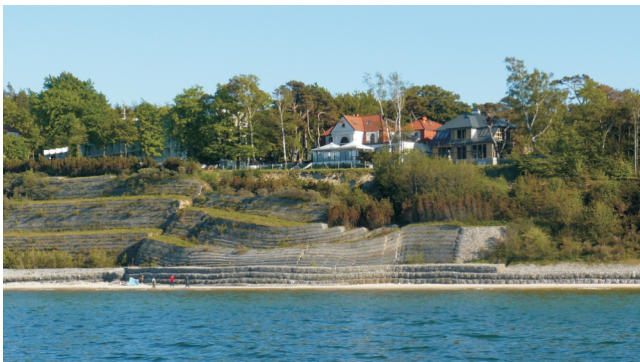
Fig. 4. Protective construction failure (phot. G. Uścińowicz)
