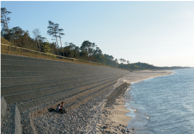
Fig. 8. Lack of beach in front of a seawall
